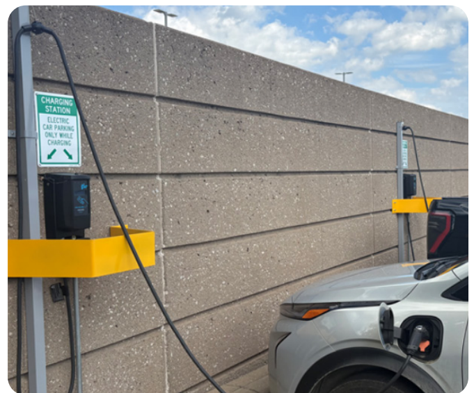
EV Chargers at MAVD.
