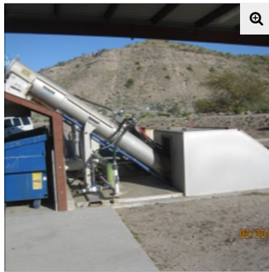
Section 18 WWTP Drum Screen
