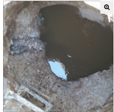
Corroded Sewer Manhole
