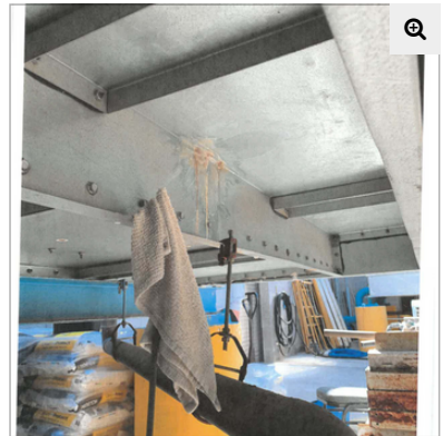
Cooling Tower #2 Before
