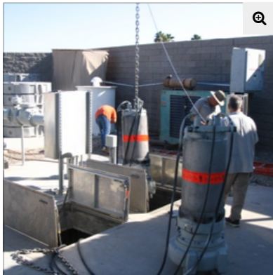
Lift Station Wet Well
