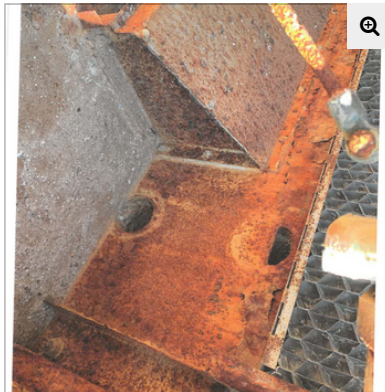
Cooling Tower #2 Before
