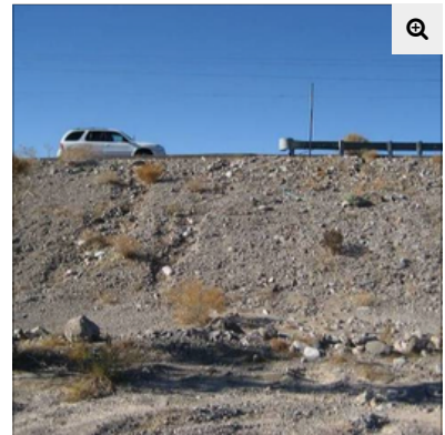
Bullhead Parkway Erosion
