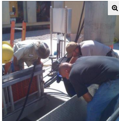
Lift Station Wet Well
