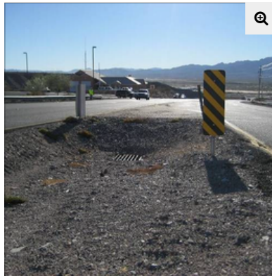
Bullhead Parkway Erosion
