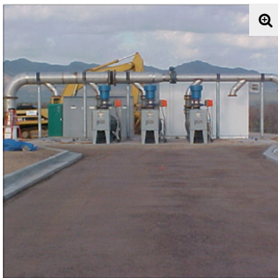
Section 10 WWTP Blowers
