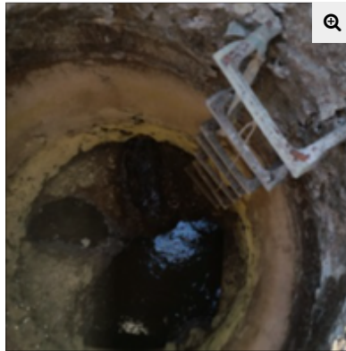
Corroded Sewer Manhole
