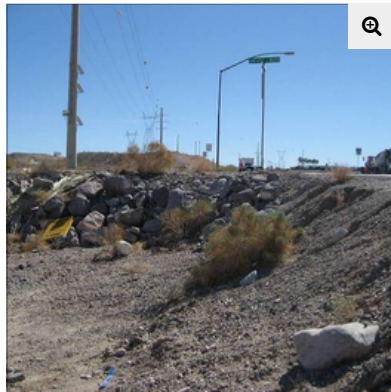
Bullhead Parkway Erosion
