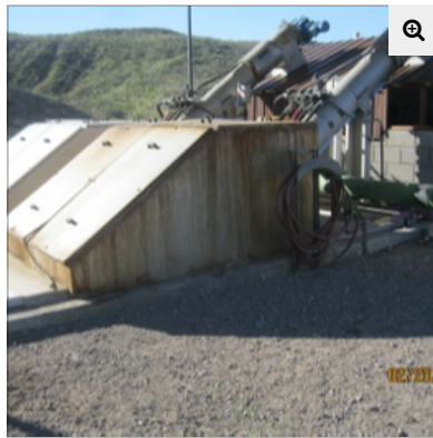
Section 18 WWTP Drum Screen
