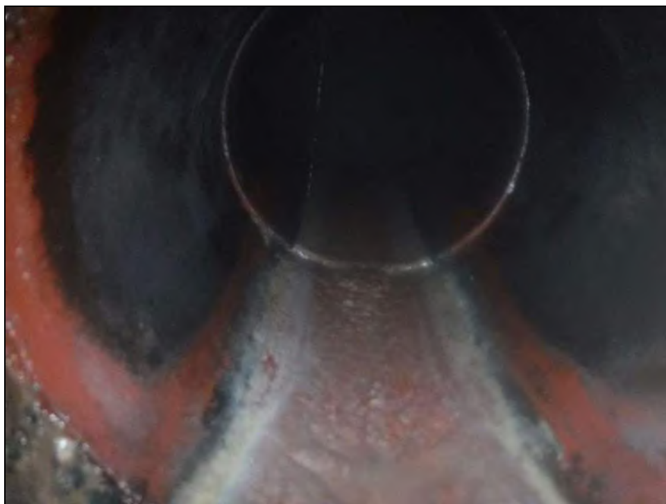
Southwest Influent Pipe
