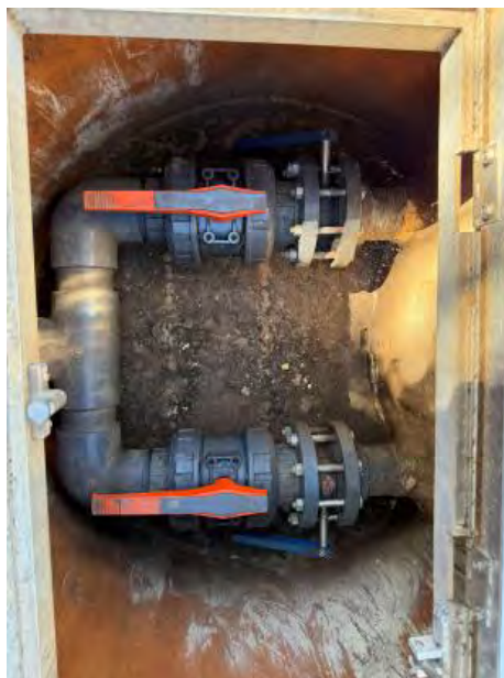
Above Ground Vault Piping
