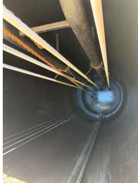
Wet Well and Piping
