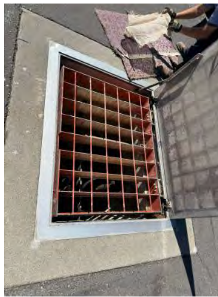
Wet Well Hatch
