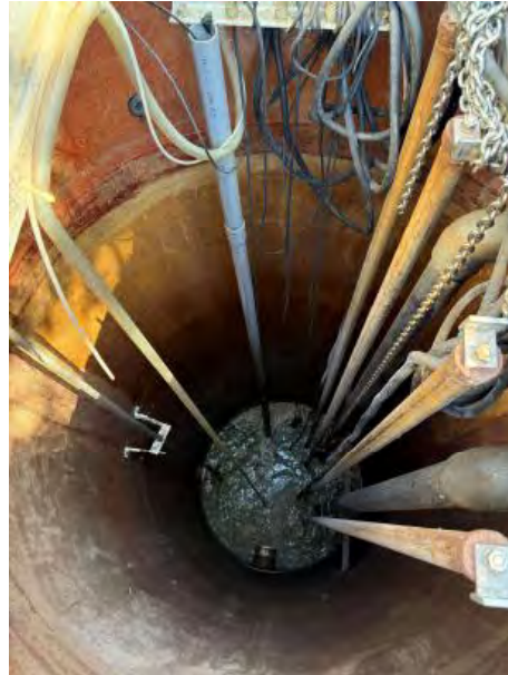
Wet Well Piping and Coating
