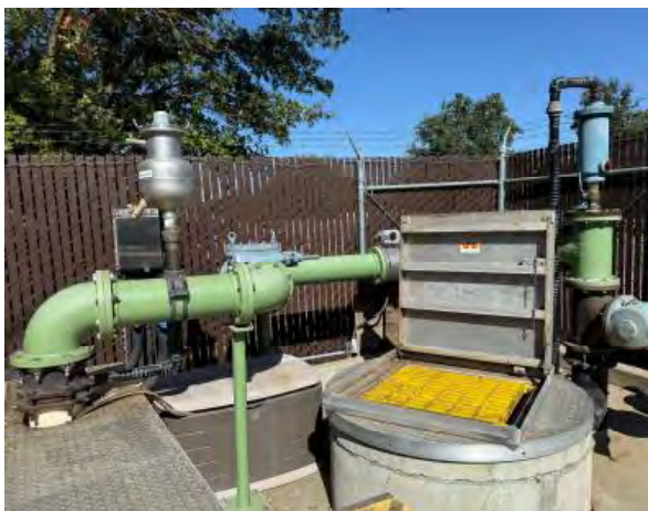
Above Ground Piping
