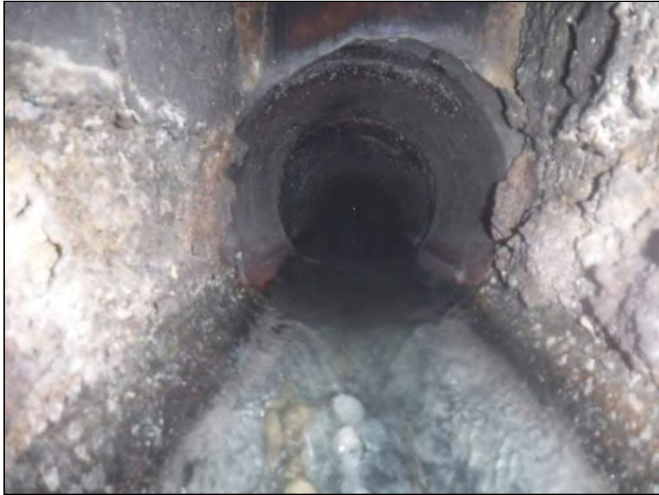
Southeast Influent Pipe
