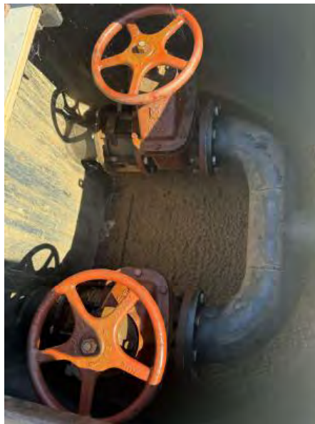
Above Grade Vault
