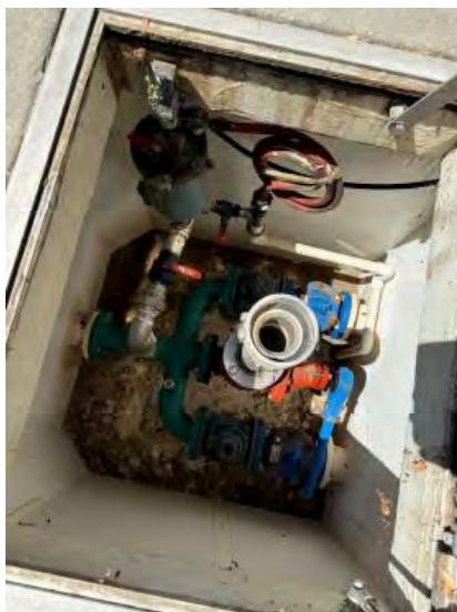
Discharge Piping Vault
